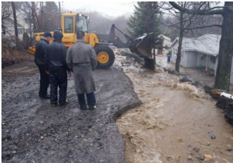
Undermining created by flooding on River Road in Tewksbury in March 2010
